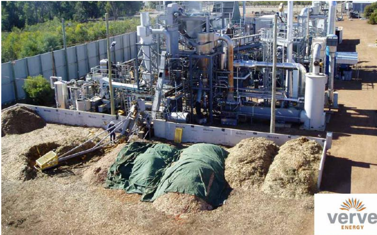
Verve Energy's Integrated Wood Processing 1MW demonstration plant.
